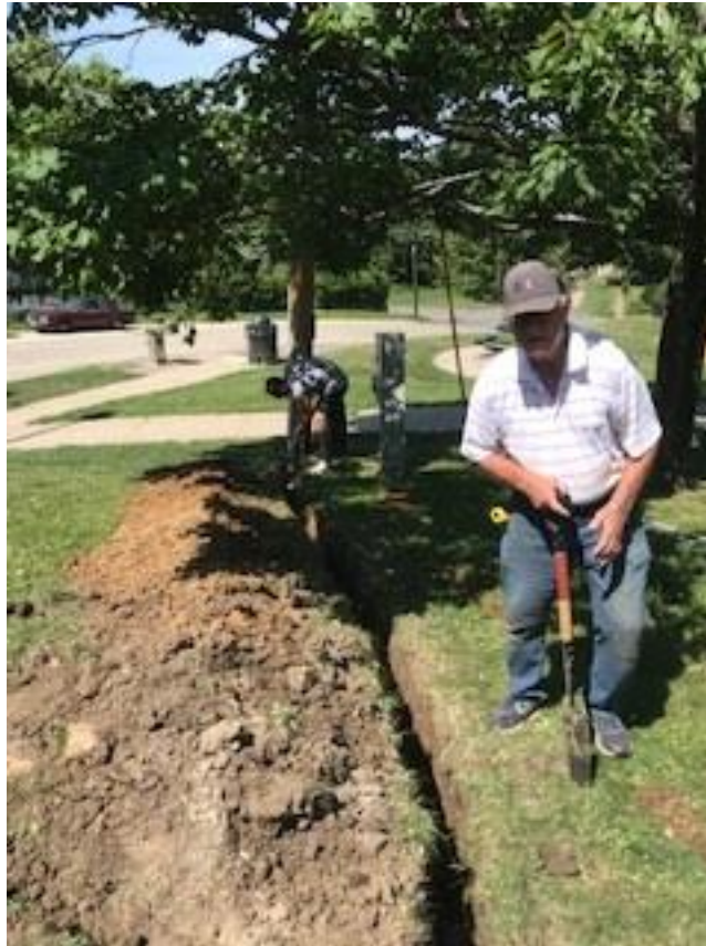
Ethan Baltz and Roger Johnson working on the lighting project behind the church.
